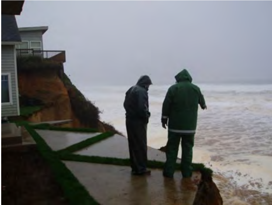
Figure 32. Bluff Failure Due to Toe Erosion by Ocean Waves
