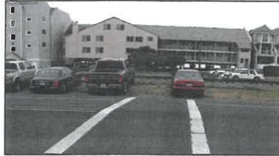
Lack of curb and gutter in southbound direction in downtown Rockaway Beach
