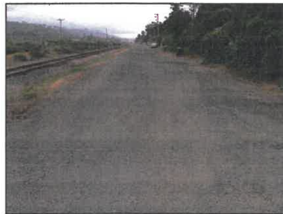
Rough chip seal makes bicycling difficult along Miller Street
