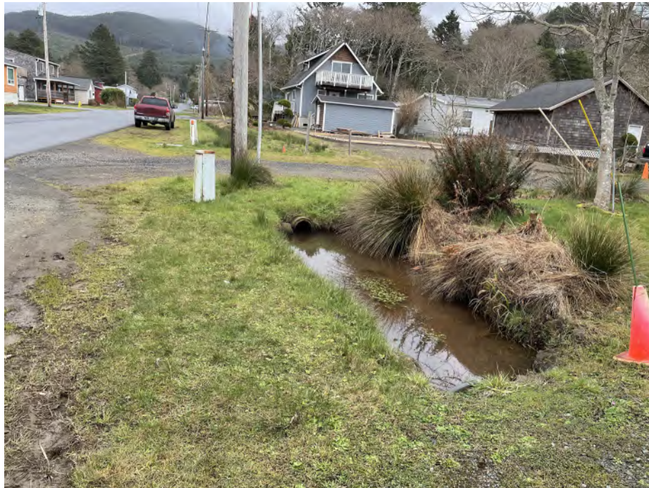
Figure 4 – Drainage Ditch on the South Side of the S 2 nd Ave & S Coral St Intersection
