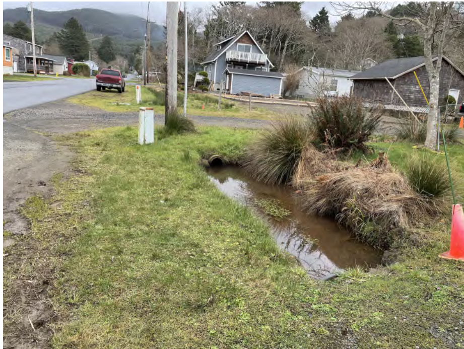
Figure 4 – Drainage Ditch on the South Side of the S 2 nd Ave & S Coral St Intersection
