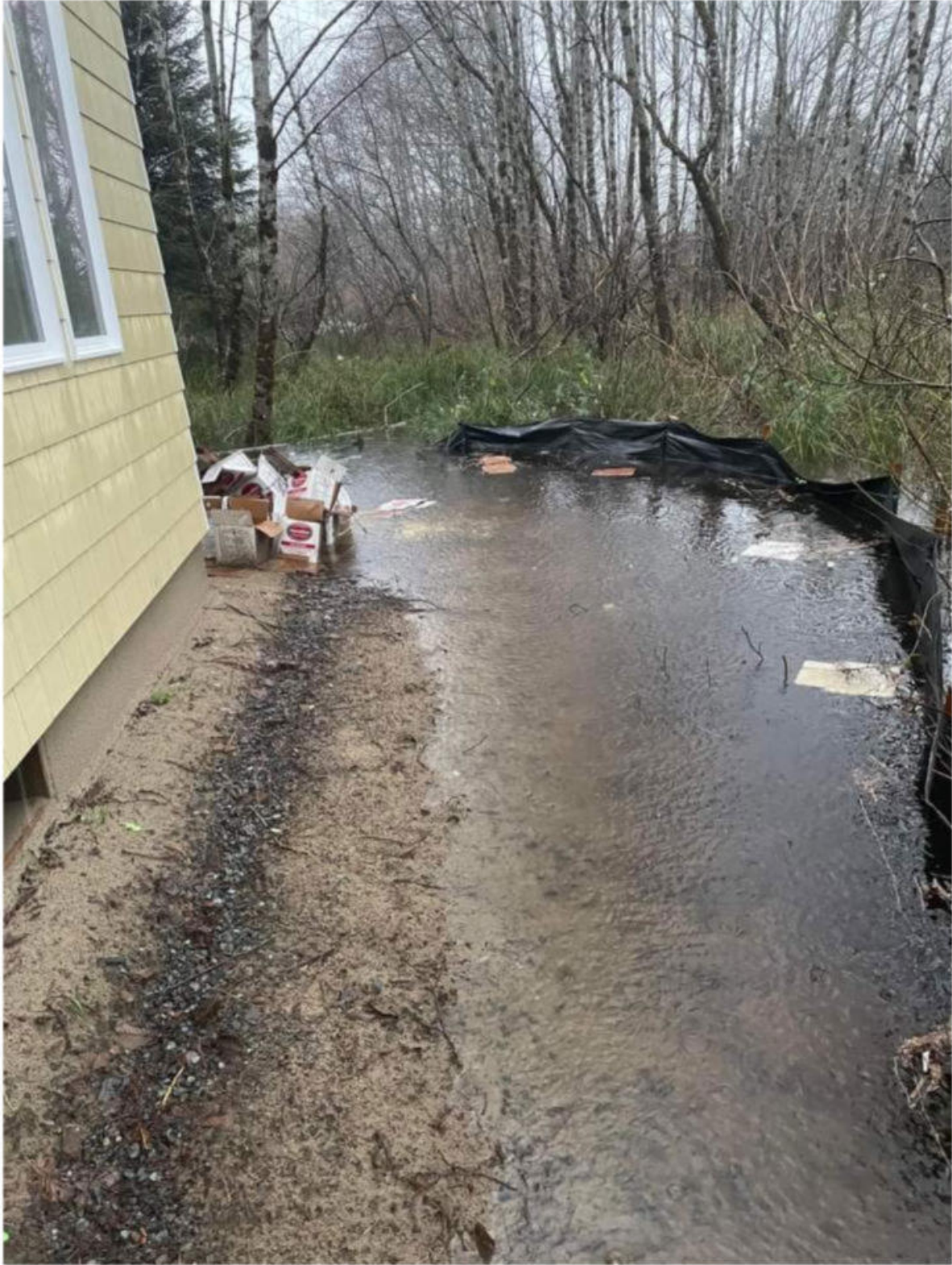
Side yard of house on SectionLine Rd 01/22 Water already in crawl space.
