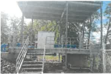
Oakland Raw Water Intake
