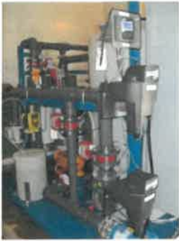
Water Treatment Plant Timber, OR
